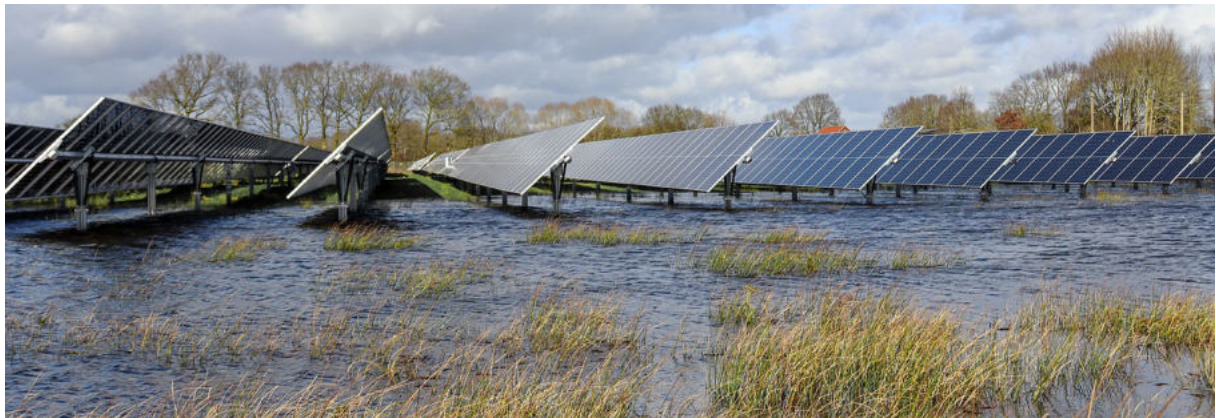
Wattmanufactur - Solarpark Lottorf ( https://wattmanufactur.de/moor-pv.html )
